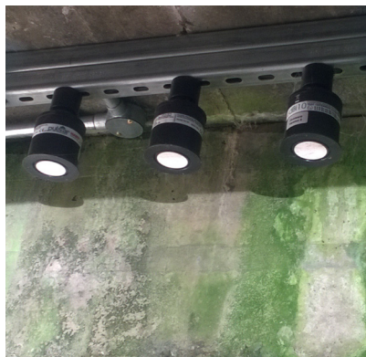
3 dBi HART transducers Monitoring Sluice Levels
